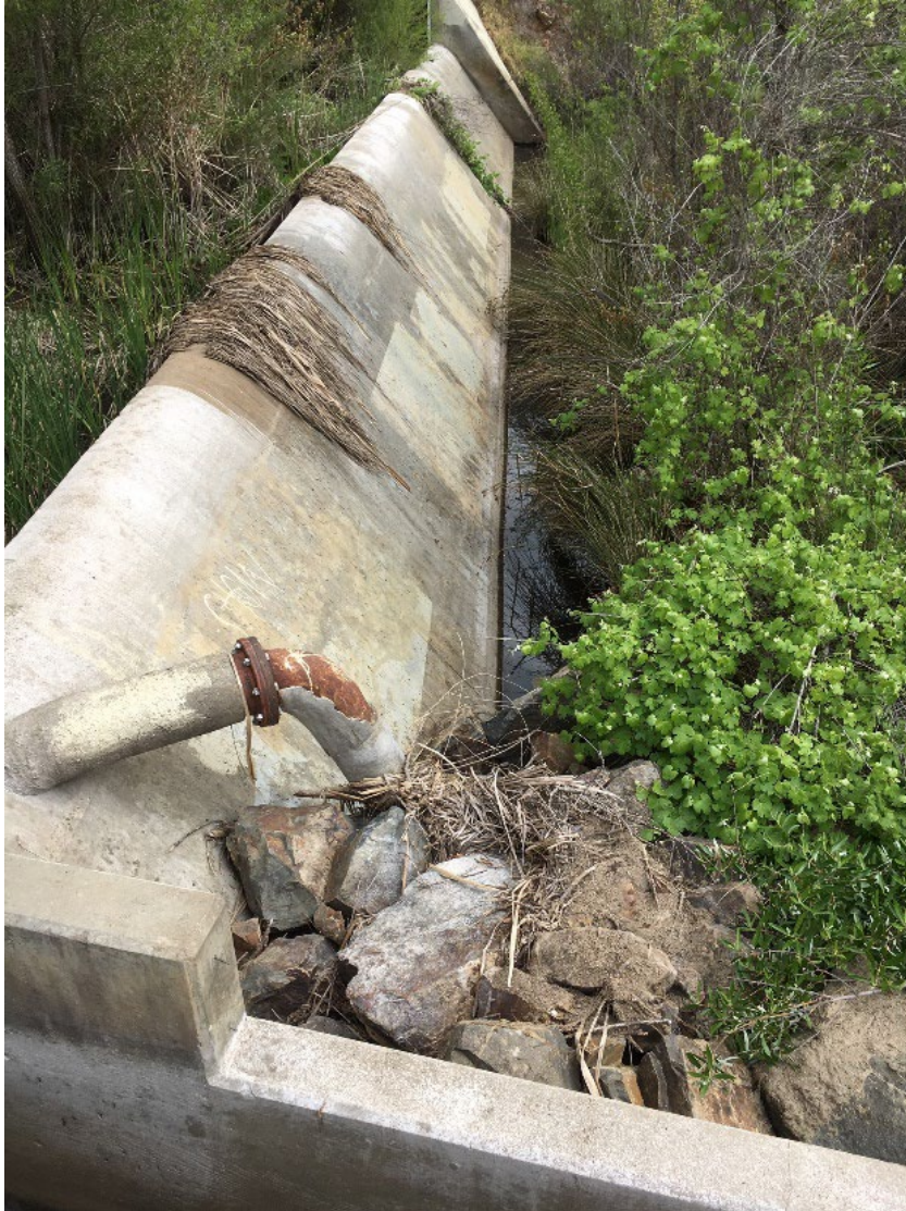
Figure HYD1.1. Example of a water diversion on the Sweetwater River (photo by C. Brown, USGS). Water diversions can impact downstream water availability and alter the stream morphology by retaining sediments.
