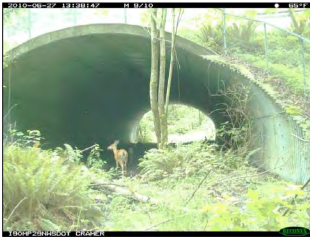
Figure 32. Example of a Class 3 Large Underpass arch culvert being used by mule deer under I-90 Washington © P. Cramer, J. Kintsch & WSDOT
