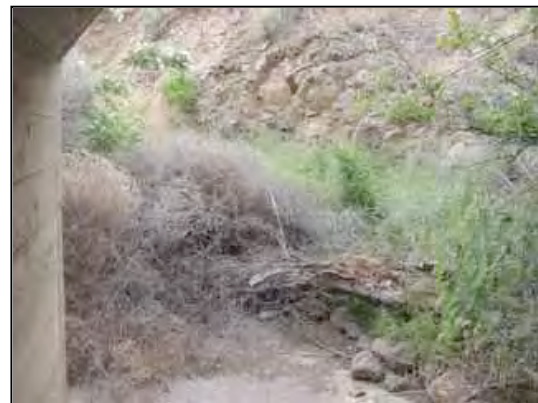
Figure 65. Debris at culvert outlet
