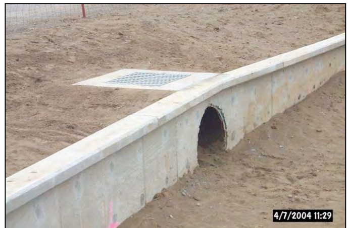
Figure 11. Turtle culvert, wall, and grate ©Port of Portland
