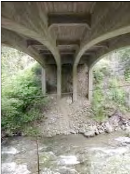
Figure 59. Steep bank on west side
