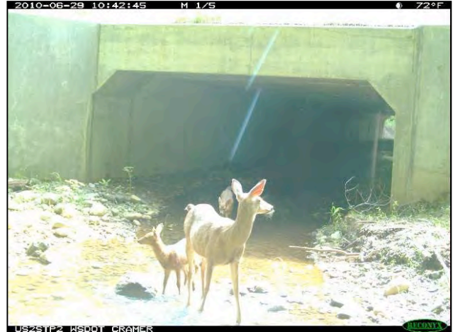
Figure 4. Concrete culvert under US 101 in Washington with black-tailed deer doe and fawns © P. Cramer, J. Kintsch, & WSDOT
