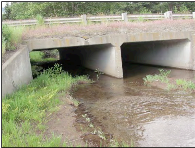
Figure 30. Example of a Class 2 Medium Culvert, I-90 WA © J. Kintsch & P. Cramer
