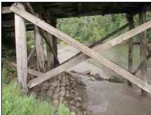
Figure 22 . Bank under structure on north side
