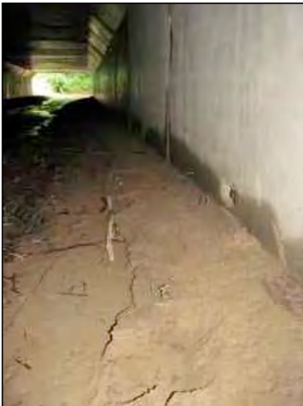
Figure 3. Muddy pathway through culvert
