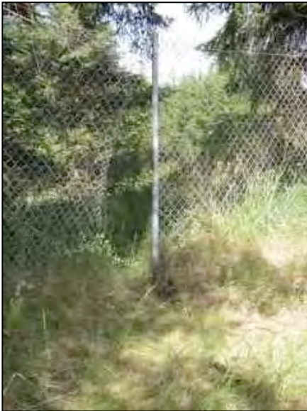
Figure 110. Gap in chain link fencing on south side
