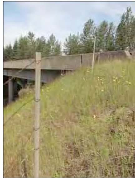
Figure 111. Large gap in barbed wire fencing through median
