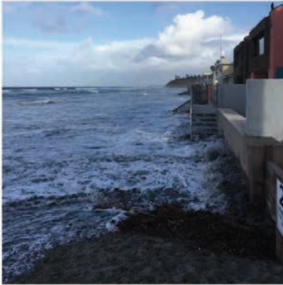
Overtopping in Del Mar, 3/8/16
