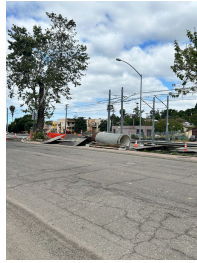
Figure 3. Safety hazard from construction material on the median at the intersection of 65th St. & Imperial Ave.
