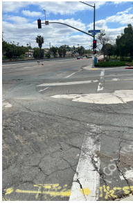
Figure 2. Crosswalks at the intersection of Imperial Ave. & Woodman St. needs repainting
