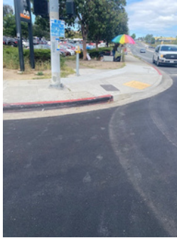
Figure 3. Needs additional curb cut (SW and SE corners of Euclid Ave./Market St.)
