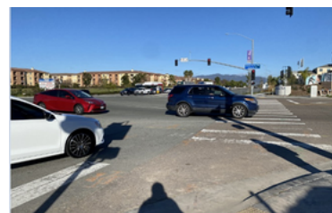
Figure 3. Crosswalks on intersection between Caliente Ave. & Otay Mesa Rd. need to be repainted.
