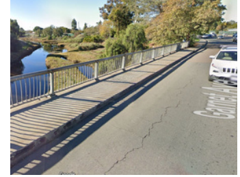
Figure 6. Narrow sidewalk on Rose Creek bridge
