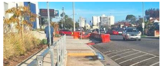
Figure 2. Handicap ramp needs repair in front of Central Elementary on Orange Ave. between 37th St. & 39th St.
