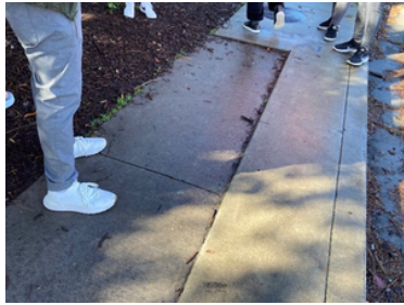
Figure 4. Lifted sidewalks along Naples St. between Broadway & Industrial Blvd.
