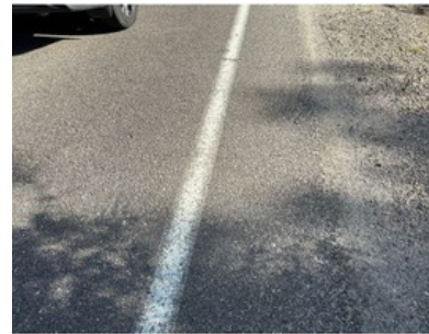
Figure 4. shows the shoulder of the road where pedestrians can walk while cars travel past with a posted speed limit of 45 mph.
